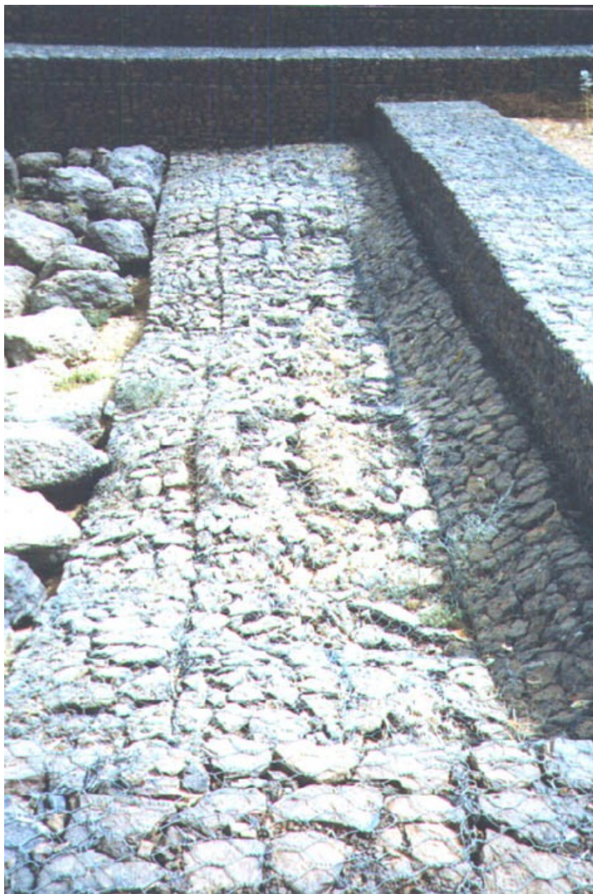
Fig. 4.28 – Damages in the gabions
