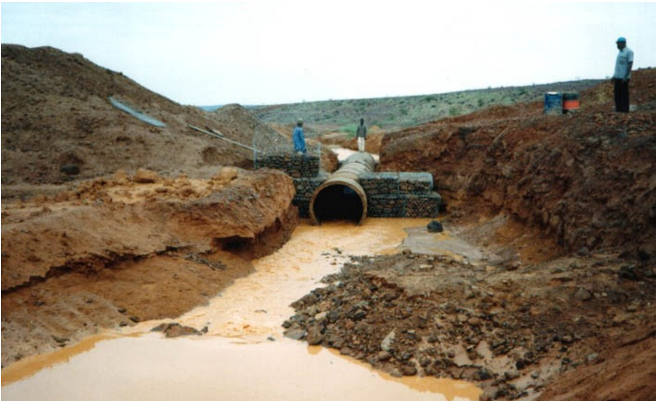
Fig. 4.2 – Runoff passing through a pipeline inserted in the earthfill during embankment construction (Akala I, Keita, Rep. Of Niger, 1990).
