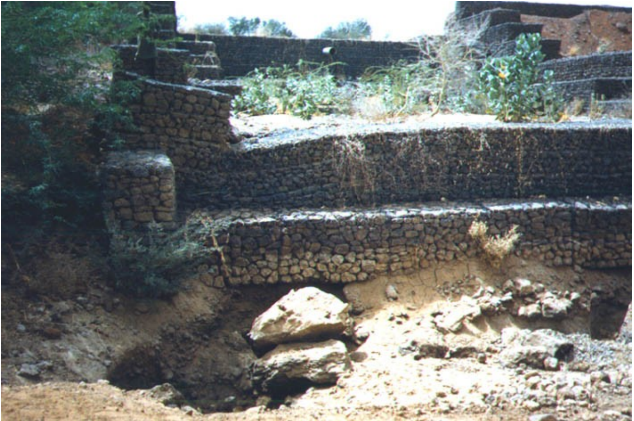
Fig. 5.6 – Damaged gabions structure without settlement
