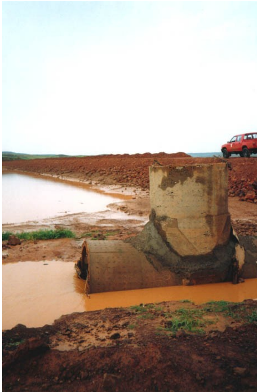
Fig. 5.8 – Pipeline in the earthfill for the evacuation of sediments from the impoundment.
